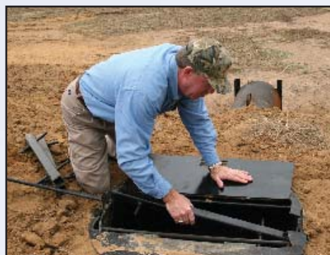
David Fowlkes inserts boards into a water control structure.
